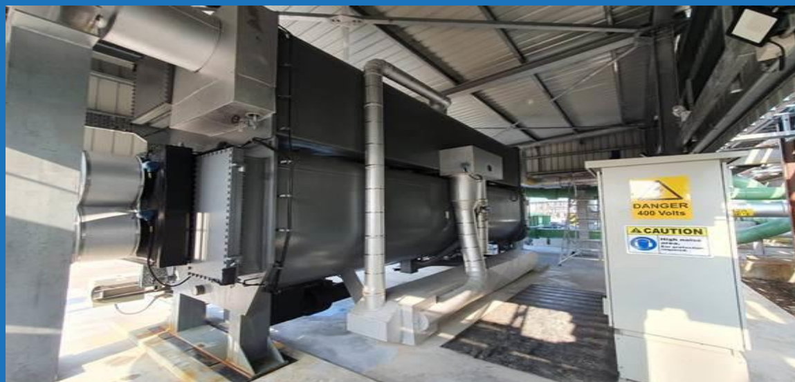
Figure 3: Seawater cooled absorption chiller
