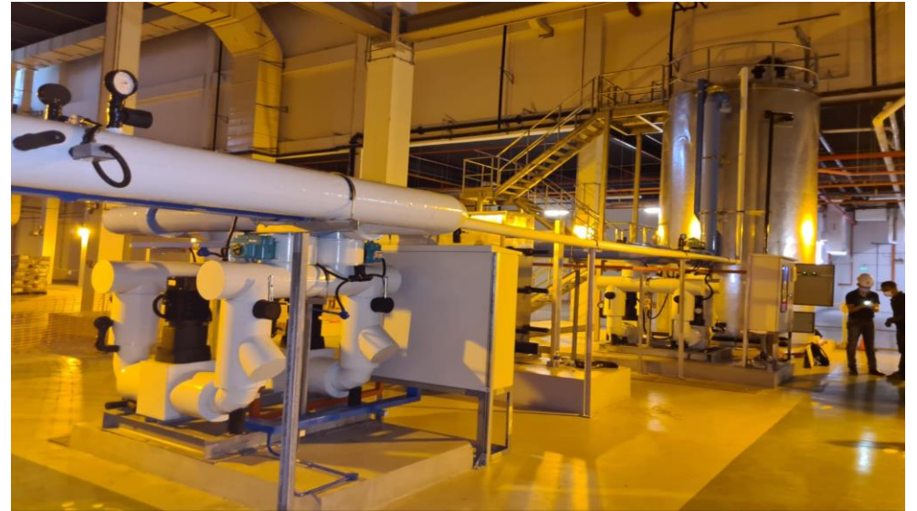
Pilot-scale PCM LTES integrated into DCS @ Keppel DHCS
