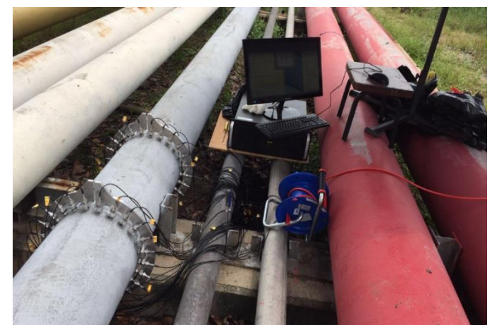
Thickness mapping on a 10 mm thick pipeline carrying Carbon Monoxide at Jurong Island.
