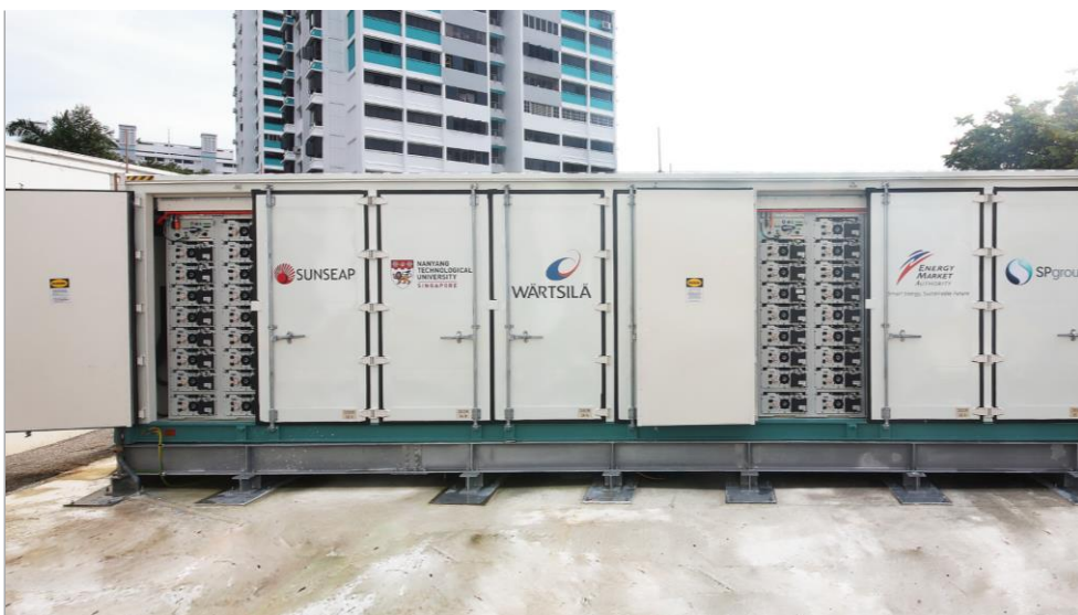
View of Battery Enclosure in the customised 40-foot container with battery racks and compartments for electrical and fire suppression devices. Externally accessible during operation and maintenance.
