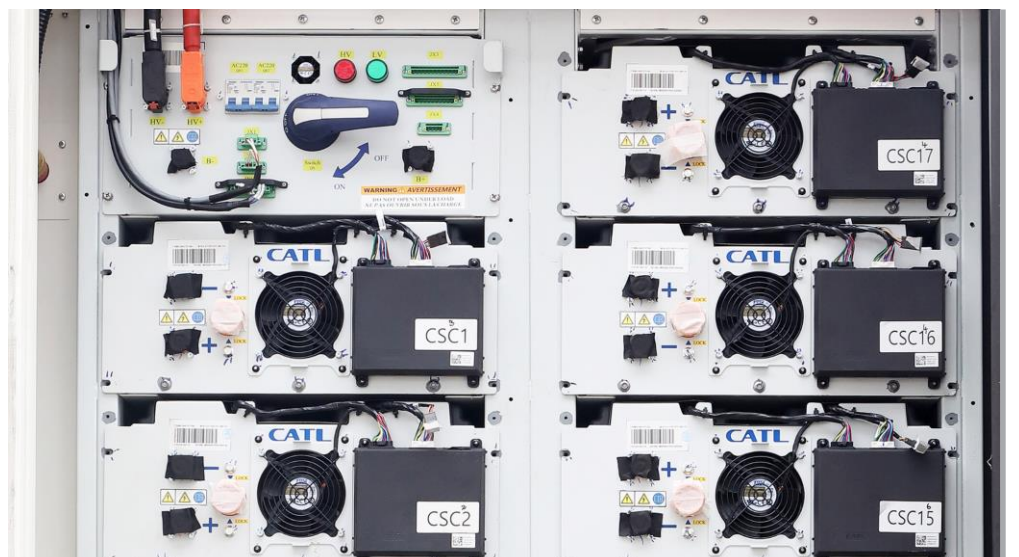
Close-up of the CATL's Lithium Iron Phosphate (LFP) battery modules.
