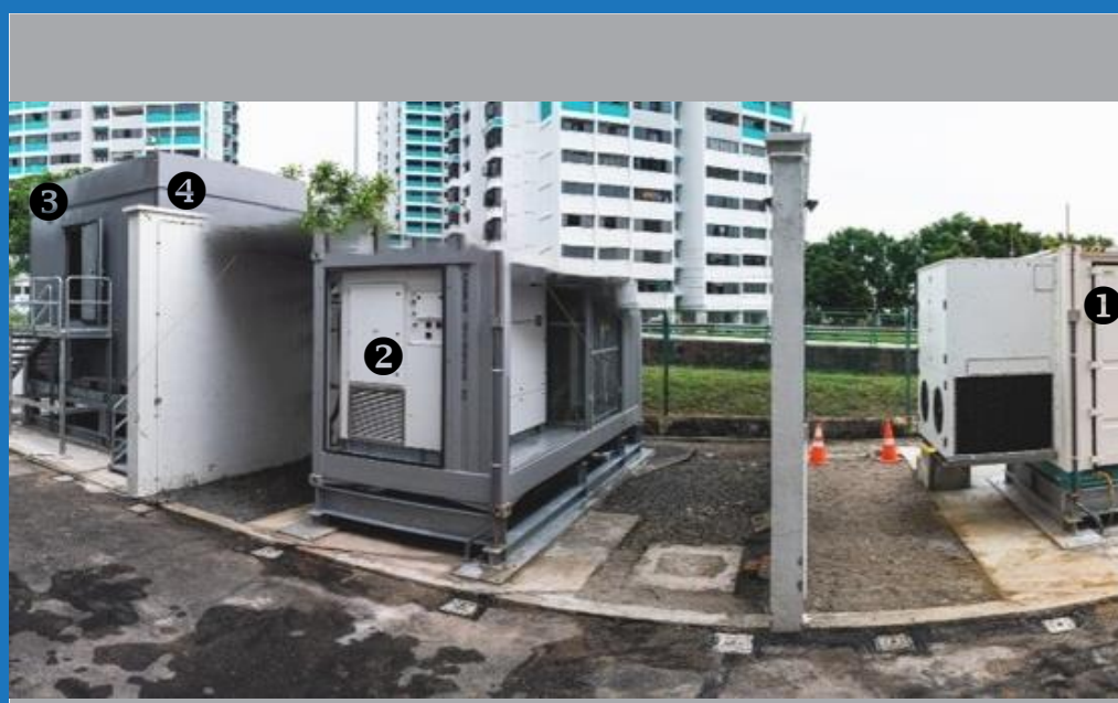
View of Battery Enclosure 1, MVPS 2, E-house with 22kV Switchgear 3 and Auxiliary Transformer 4.
